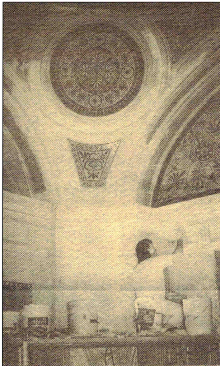
Paul Browning of the Pymer Plastering Company is shown undertaking a delicate and time consuming task of replacing sections of damaged decorative plaster. Molds made from the original pieces have been used to ensure replication.
